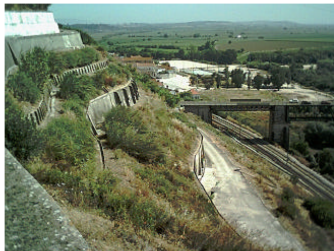
Fig. 2. Slide prevention workings built at the Santarem slope, with railway and Tejo river at the right side
